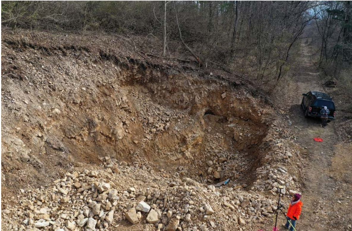
Photograph 1: View looking easterly at the conclusion of the limited 2022 Machine-Assisted Geologic Exploration of the Westerly (Upper) Wavellite Adit/Pit. Previously existing spoils that were used to build up and berm the road. New spoils that do contain specimens of wavellite overlooked during the exploration. The active workings extend below the cardboard box easterly into the wall. The westerly side of the pit contains no wavellite. Wavellite extends from the lower left (westerly, exposed) shoulder of the excavation to 3 feet off the southerly wall (road), down about 16 feet and easterly toward the easterly pit.
