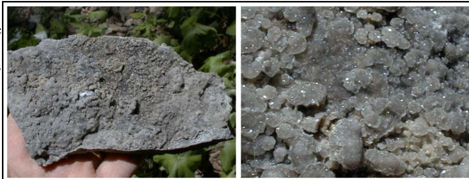
Figure 3. Encrusting crystalline gypsum on limestone surface, closeup right.
